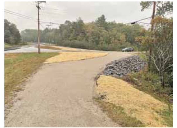
FNRT Director Ricker Miller headed up the 2022 Recreational Trails Program grant project at the Plains Road intersection of the Northern Rail Trail and busy New Hampshire Route 11 in Andover. The project addresses safety and visibility issues.
